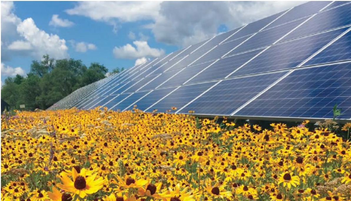
Solar panels in the Hudson Valley, New York. Photo: Scenic Hudson
